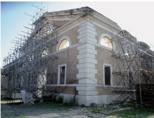
Fig. 6: The temporary constructions to stabilise structures and to ensure safety in the building site. © Anna Raimondi.
